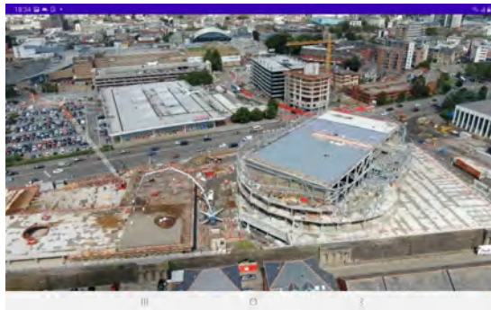
Figure 6.4: A snapshot from the drone footage taken above the arena. The footage from which this snapshot is taken begins from the location of the installation and travels across the top of the development site before completing a 360 degree tour of the arena.
